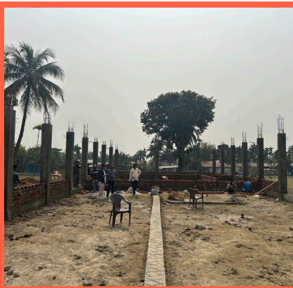
Er. Tahsin Khan on inspection visit at construction site of Flood Shelter at Kathoni, Morigaon
